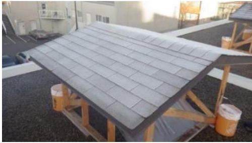
Figure 2.12 – Frost on exterior of shingles during morning of January 2, 2013
