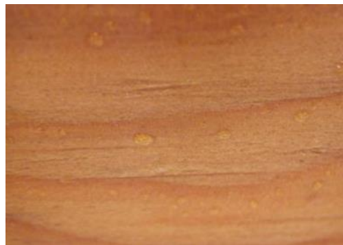
Figure 2.15 – Condensation on underside of plywood sheathing on morning of January 2, 2013. Note that surface condensation at this time is only visible on certain areas of the plywood and was affected by wood grain.
