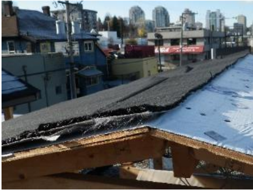
Figure 1.15 New vented drain-mat layer installed over the existing self-adhered membrane in the control roof
