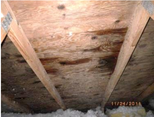
Figure 1.1 Visibly wet roof sheathing caused by rainwater ingress through the shingles and underlay
