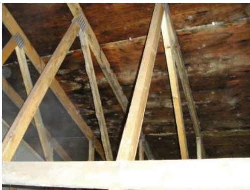
Figure 1.3 Widespread stained, wet, and deteriorated sheathing within wood-frame attic from persistent indoor and exhaust duct air leakage and poor attic ventilation
