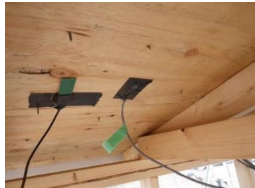
Figure 1.23 – Condensation sensor and surface temperature sensors installed in March 2013 to interior side of sheathing
