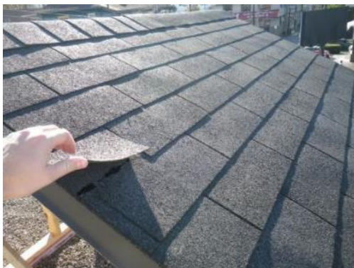
Figure 2.24 – Poor self-sealing at majority of shingle tabs on North slope observed for several months after installation.
