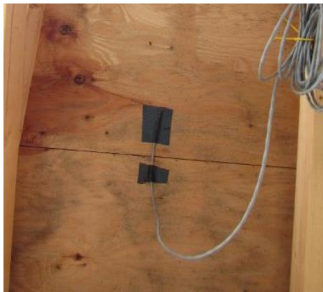
Figure 2.9 Fungal growth on the underside of the North orientation of the 4:12 roof including two areas with surface treatments which are discussed in later section of this report
