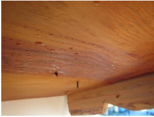
Figure 2.16 - Condensation on the underside of the roof sheathing on October 3, 2013 showing a location where it has been absorbed by the sapwood but has not been absorbed by the heartwood.
