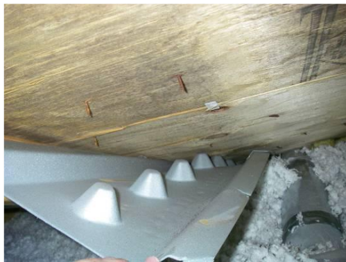
Figure 1.4 Fungal growth on sheathing within the ventilation baffles as a result of the entrainment of humid, outdoor air
