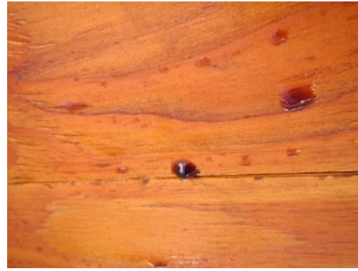
Figure 2.17 - Condensation on the underside of the roof sheathing on October 3, 2013 showing a location where extractives from the wood sheathing are visibly noticeable in the condensation droplets
