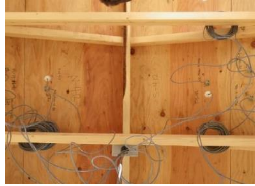
Figure 1.19 – View of underside of 4:12 roof hut showing placement of moisture pins and sheathing temperature sensors
