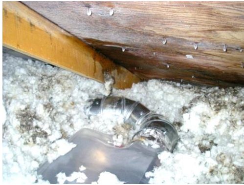
Figure 1.2 Locally stained and wet sheathing due to condensation (frost) of humid air which is leaking from a poorly sealed bathroom exhaust duct
