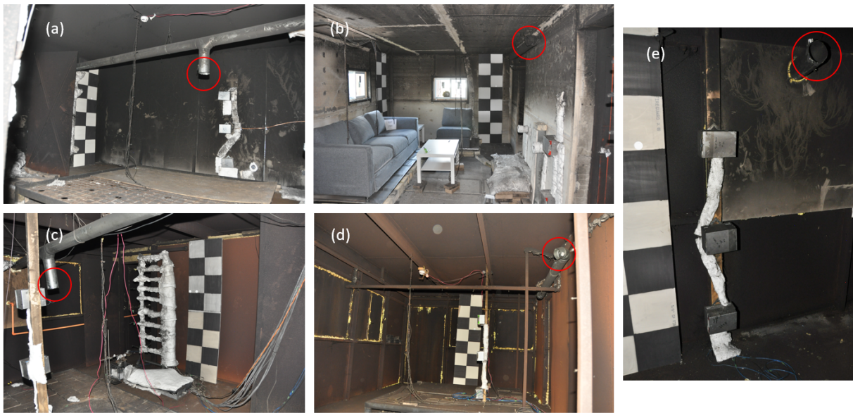
Figure 5: Images of HVAC vent locations at (a) first floor SW room, (b) fire room, (c) second floor SW room, (d) second floor SE room, and (e) second floor exhaust.
