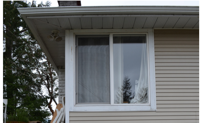
A window located on a facade with low rain exposure, protected by a large overhang.
