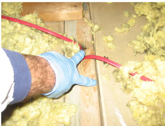
Air sealing of an electrical penetration and unsealed top-plate connection in an attic.
