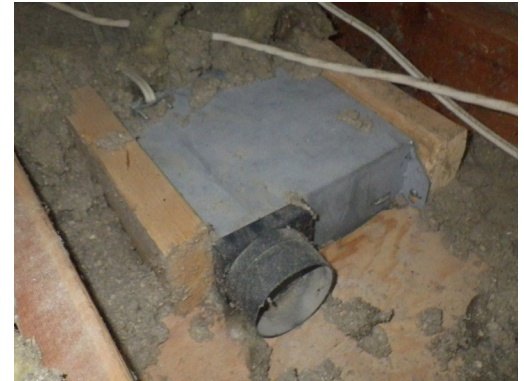
Bathroom exhaust fan venting into the attic. Conditions such as this should be remedied prior to or as part of air sealing and insulation work.
