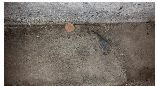
Cracks in the slab and gaps between the slab and the foundation wall.
