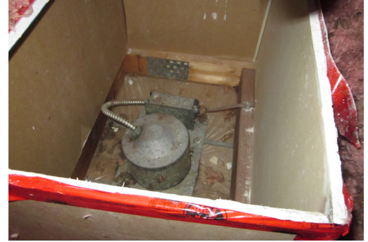
Boxing out existing non-IC-rated pot lights mitigates air leakage at these locations.
