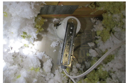
Above is an example of a poorly installed pot light where no measure of air sealing has been taken.
