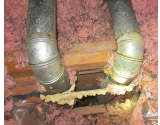
A relatively large hole in the ceiling plane through which two ducts are installed.
