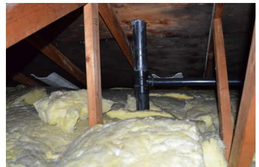
Accessible attic with potential air leakage around the plumbing stack penetration through the ceiling.
