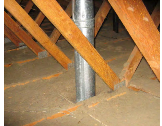
Uninsulated and un-sealed exhaust duct running through an attic, leaking air and heat to the space.
