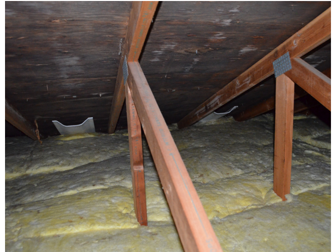
Insulation baffles installed at every second truss bay prior to installation of insulation to provide openings past the insulation from the soft vents to the attic space.
