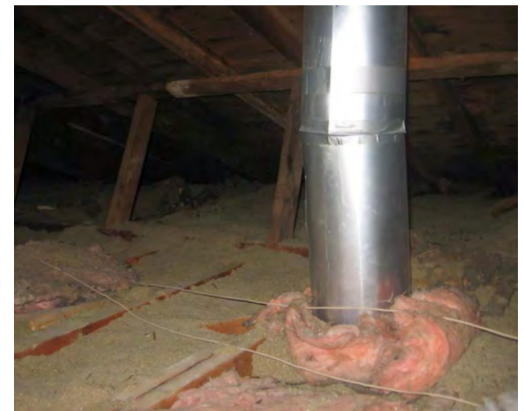
Insulated exhaust duct in attic.
