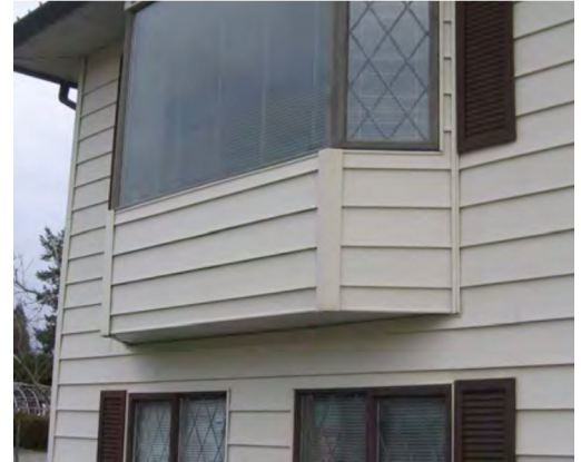
Overhanging floor under a bay window.
