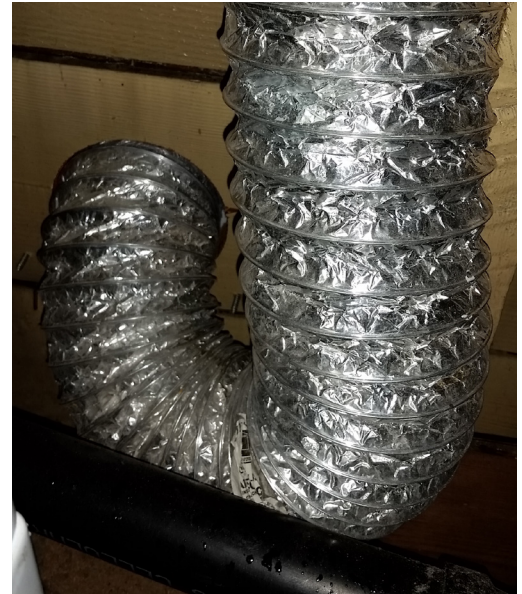
Unsealed duct penetrating the exterior wall. Duct penetrations should be airtight to avoid moist air being drawn through the wall and condensing inside the wall.
