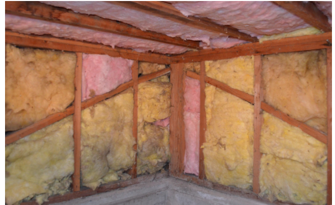
Partially finished basement/crawlspace with pony wall lacking an air barrier/vapour retarder.
