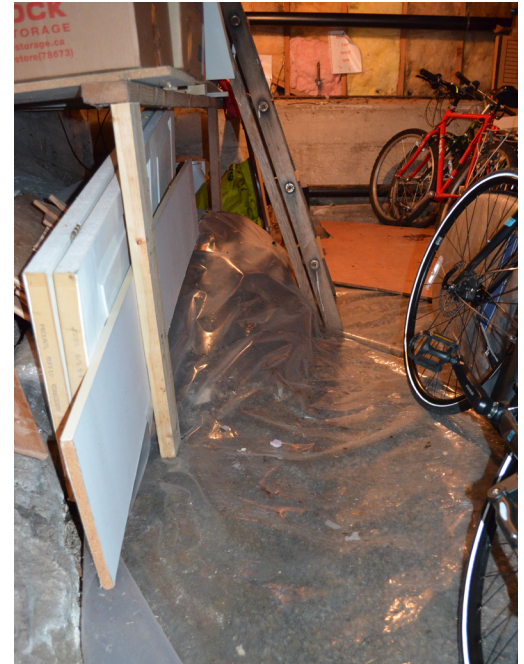
Certain floor conditions are difficult and impractical to air seal. Here a polyethylene sheet has been placed on top of the gravel and bedrock floor to reduce vapour drive into the crawlspace. The polyethylene in this frequently used basement will most likely be damaged.
