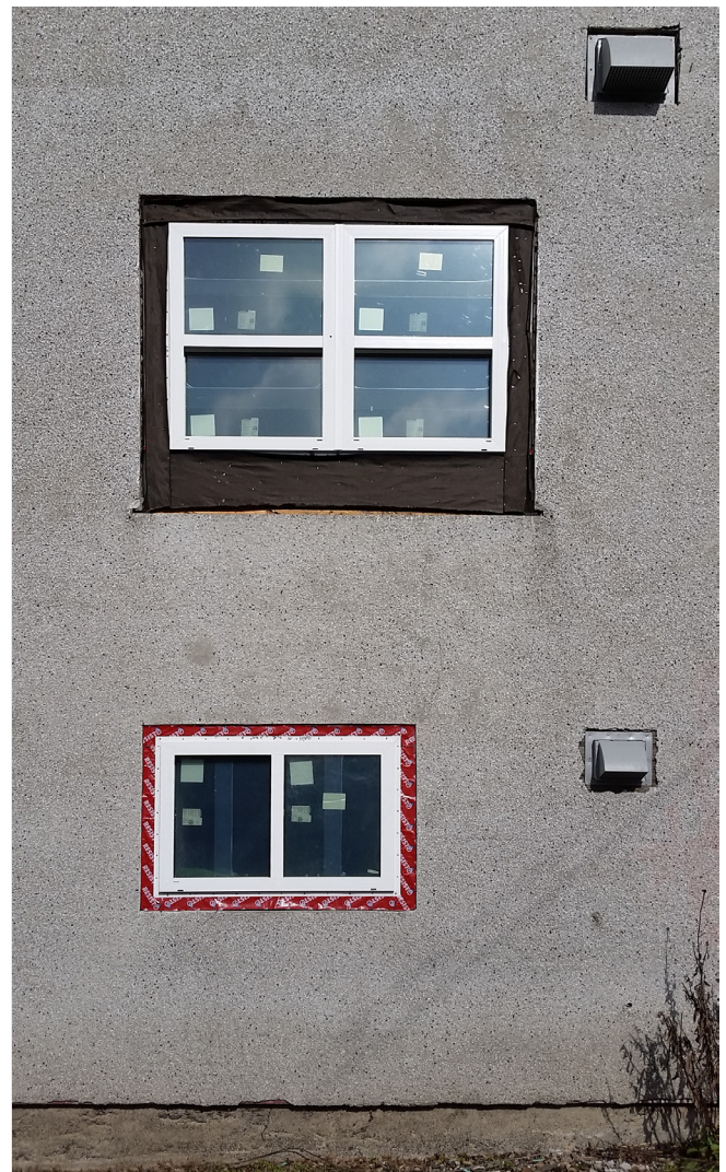
Windows being installed on a high wind- and rain-exposed facade with no overhang protection.
