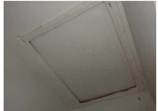
An attic access cover made from plywood resting on a wood-trimmed opening.
