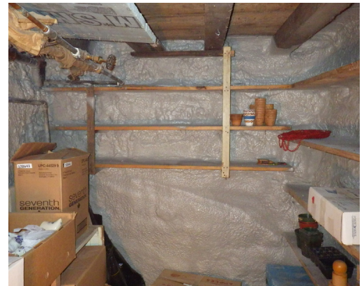
Crawlspace walls insulated with spray foam left exposed.
