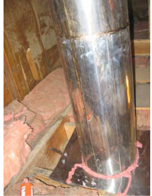
Metal chimney with sheet metal seal over ceiling joists.
