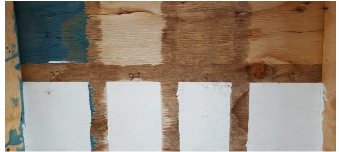
Example of surface treatments on the underside of roof sheathing showing their effect in inhibiting surface mould growth
