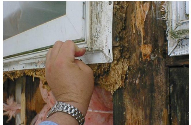
It may be desirable to replace windows and doors in cases where poor installations may have led to deterioration of the wall framing. The image above shows extensive decay visible at a window rough-opening interface detail upon removal of cladding. Damage extends well beyond window replacement work area.
