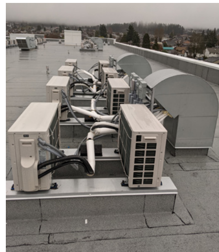
Maitland Street Village. Port Alberni - 46 units. Rooftop units
