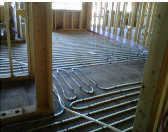
Rose Harbour. In-floor radiant heating
