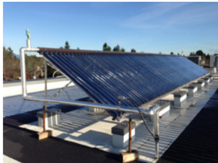
Alexander Street. 139 units - 7 storeys. Solar system re-commissioning
