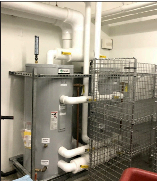
1249 Howe St. Two pre-heating storage tanks added upstream of high zone DHW tanks
