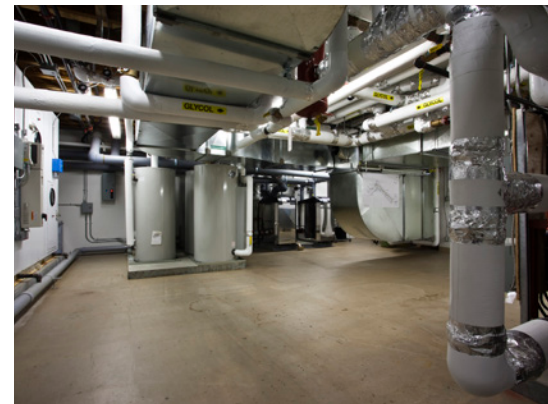
Driver House. 10612 17 St., Dawson Creek – mechanical room
