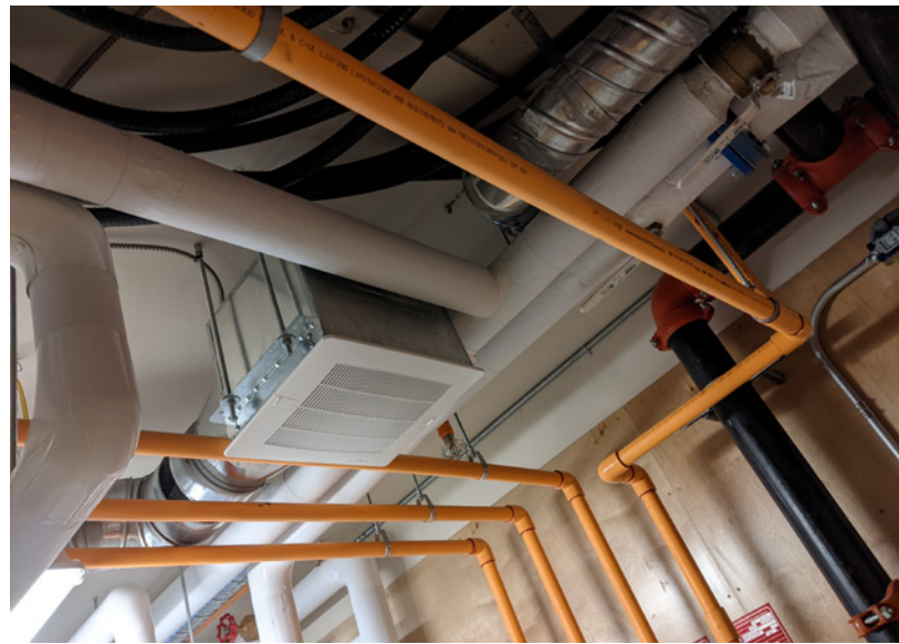
Maitland Street Village. Port Alberni - 46 units, 4-storey apartment. Fan coil unit
