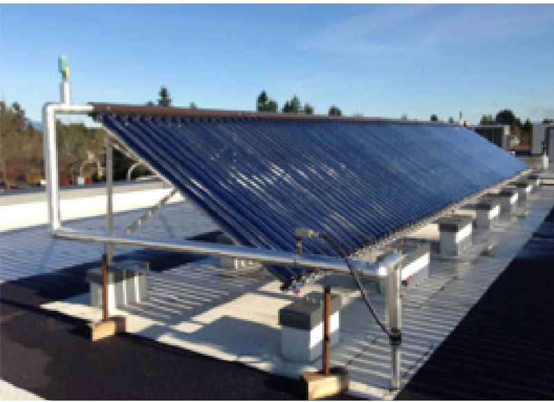
Alder Gardens. 36 units - 4-storey wood frame apartment with 1-level underground parking. Solar domestic hot water heating
