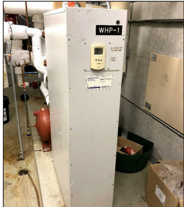
1249 Howe St. Water-to-water heat pump WHP-1
