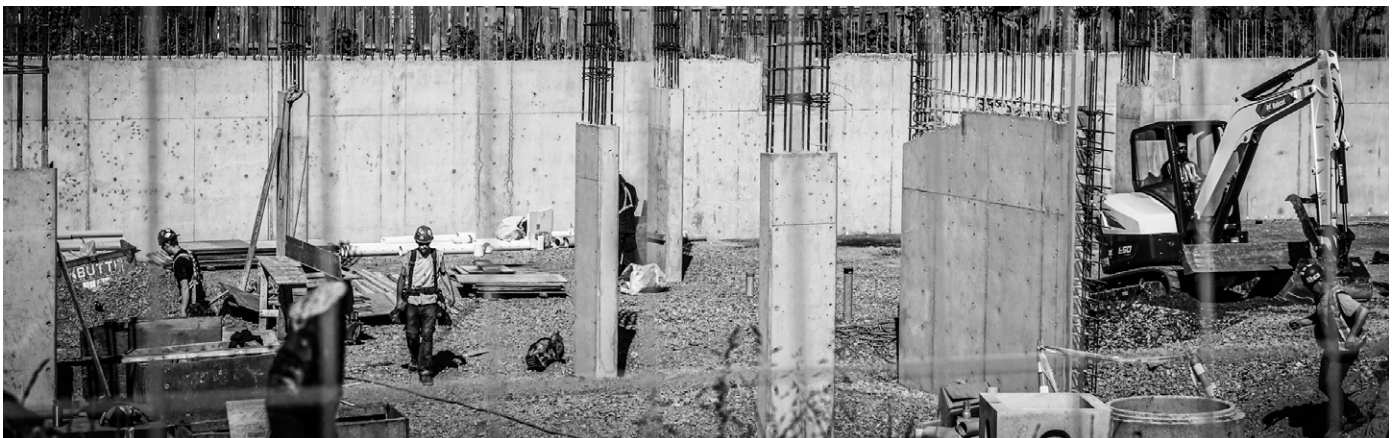
2570 Fifth St., Victoria – 60 new rental homes under construction in Victoria through the HousingHub program.
