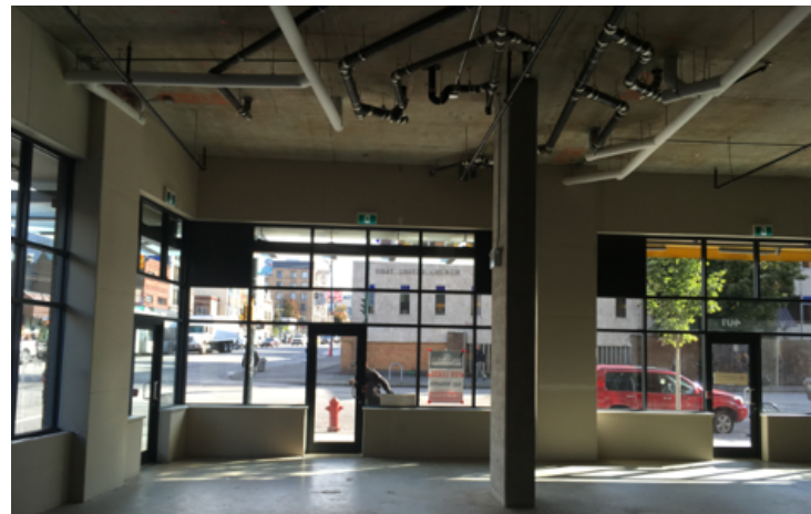
The Anjok - 298 East Hastings, Vancouver - multiple small CRUs where there is a good possibility of combination by a single tenant
