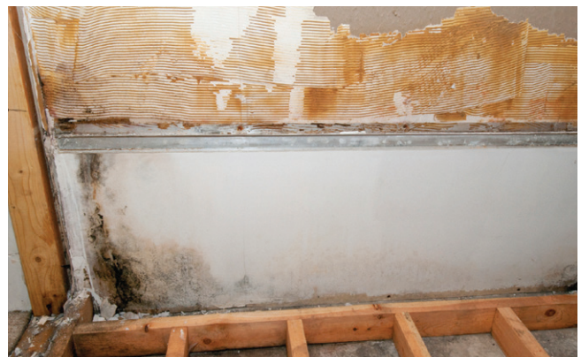
Black mould revealed during the renovation of a basement bathroom.
